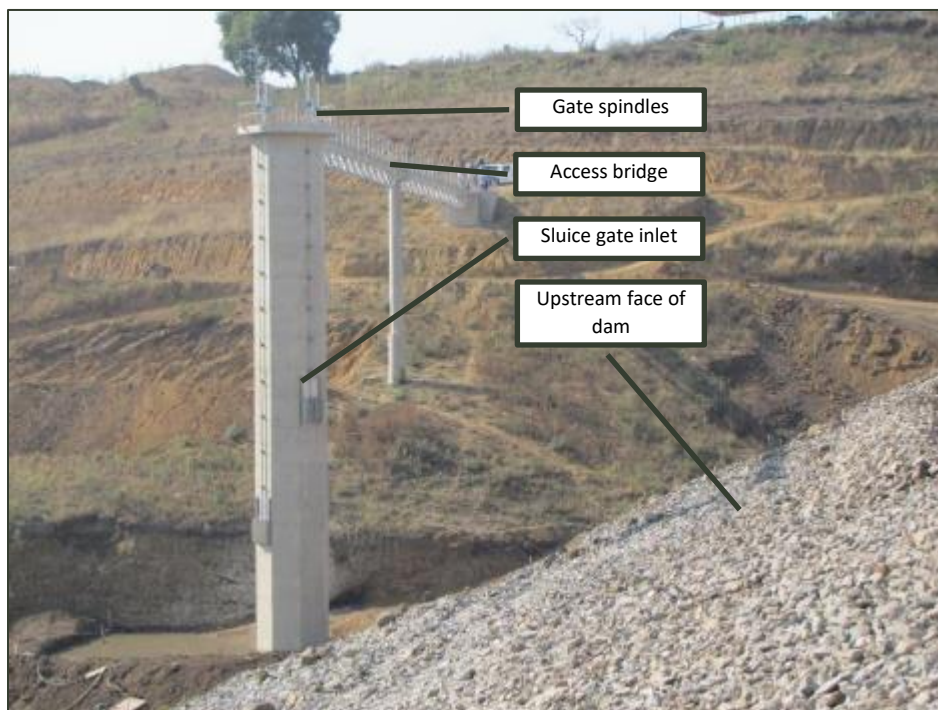
Figure 4-17 Typical wet-well outlet tower and access bridge.
