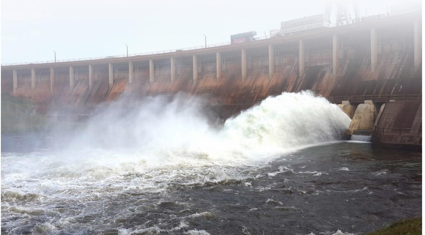
Nalubaale (Owen Falls) Dam in Jinja, Uganda. Ensuring resilience of such water sector infrastructure projects to the negative impacts of climate change is paramount
