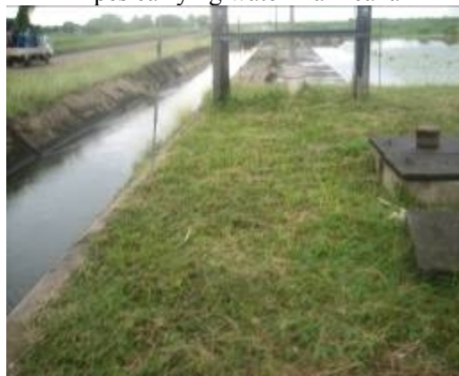
Sub-pumping station supplying water to sprinklers
