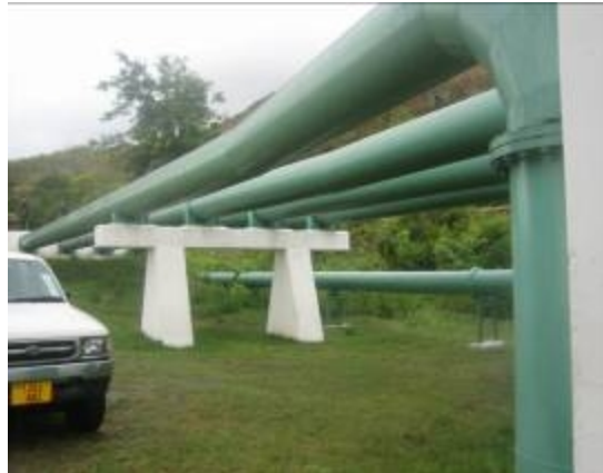
Pipes carrying water main canal
