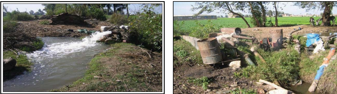
Figure 5. Private lifting Pump on old Meska (old practice)
