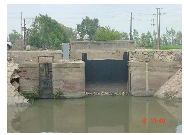
Figure 11. Old Control Gate in Branch Canals
