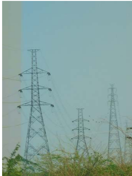
Figure 16 : 220 kV Khartoum Ring_ Nile River Crossing View
