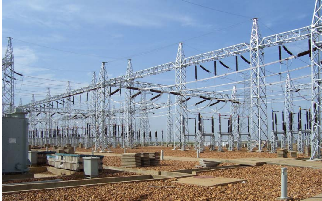
Figure 2 : Existing substation at Rabak, a similar substation will be constructed at Mandaya HPP
