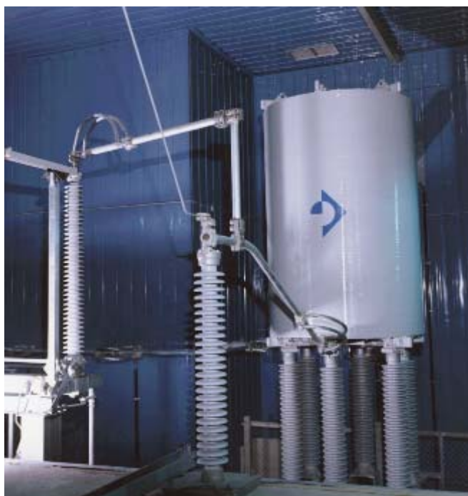
Figure 10 : Typical Smoothing Reactor
