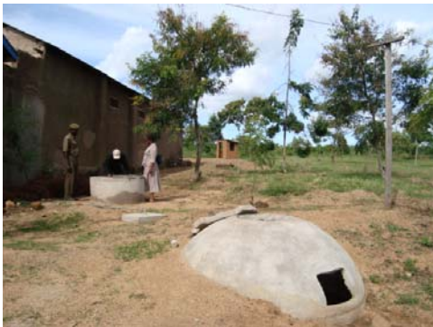
Plate (36): Biogas Unit
