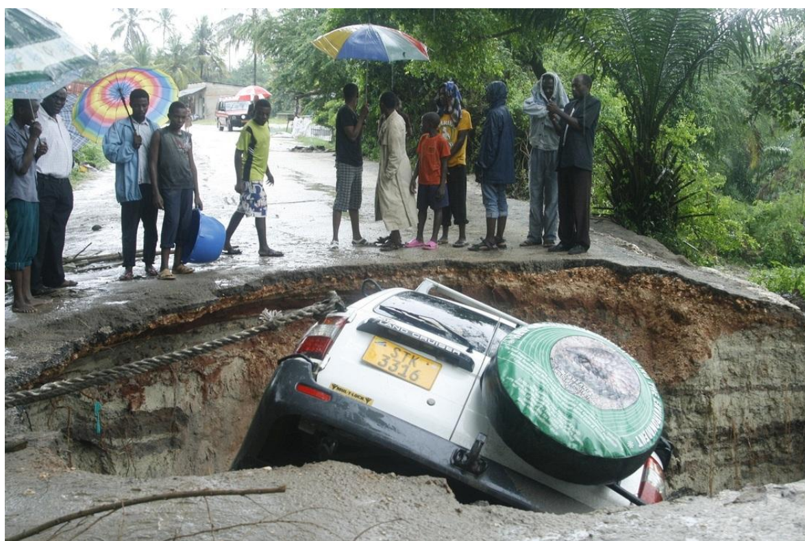
Figure 11: Road destruction by floods at Tandale Mtogole, 2011
