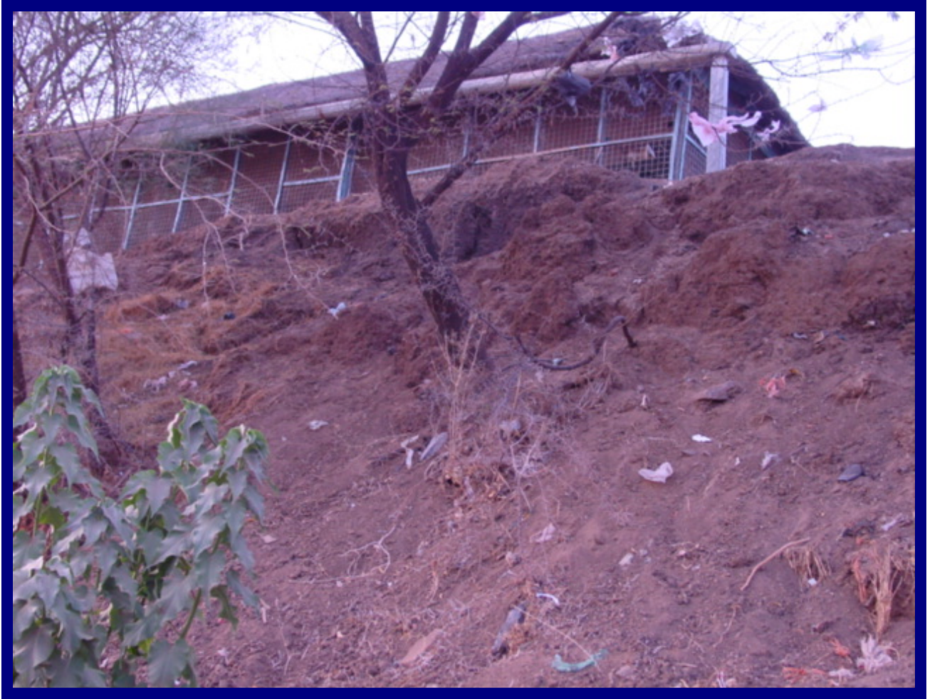
Plate No. 4: River bank erosion undermining property close to the bank (AISuki)
