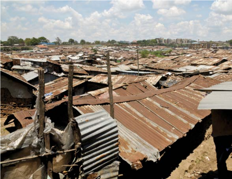
Rusting corrugated iron roofs on one of the slums of Nairobi, Kenya.
