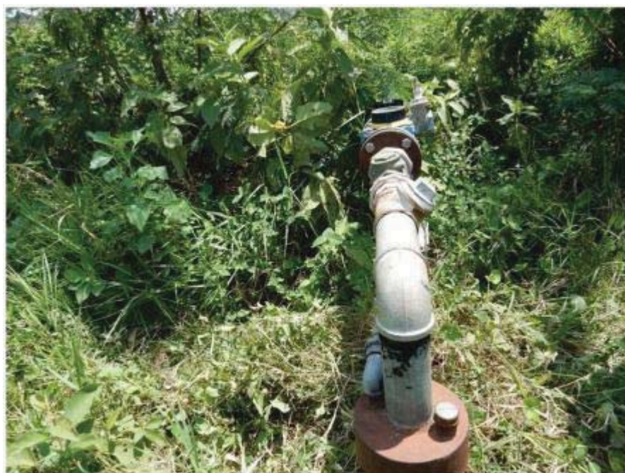
Groundwater Level Monitoring Station at a Production well at Kisumu Port Compound
