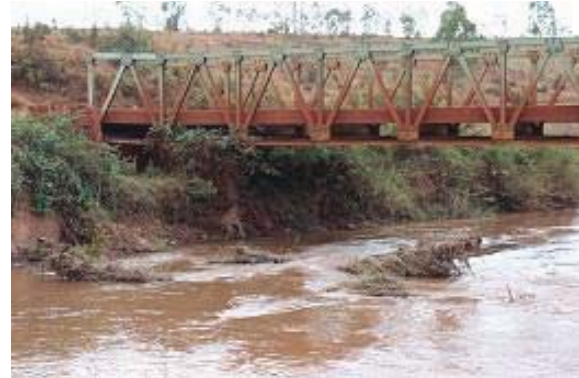
Remnants of the old steel bridge obstructing river flow at the control section
