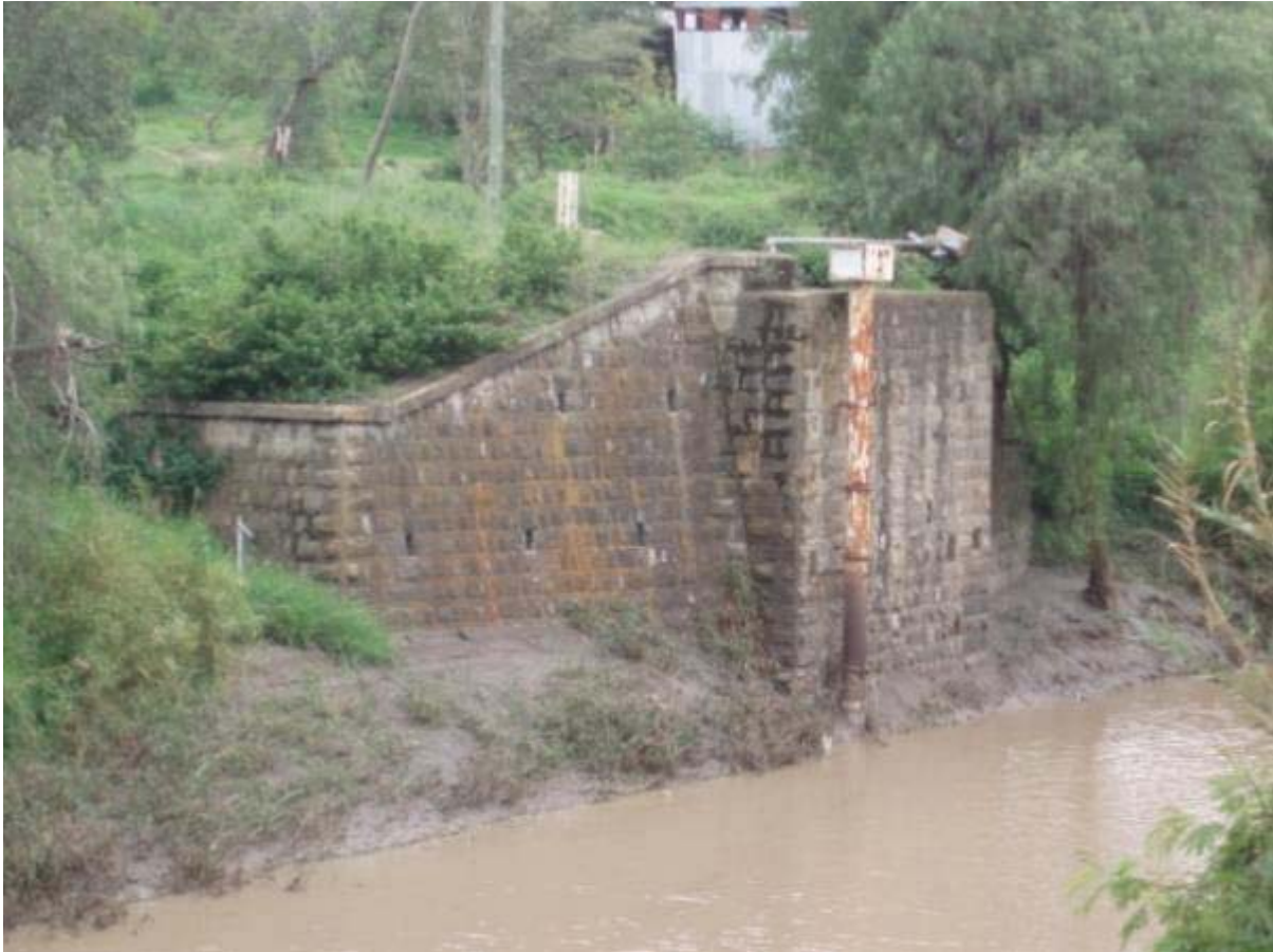
Stilling well used as mounting for radar sensor; former support for cableway in background top center; staff gauge left center
