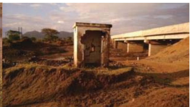
Old Grumeti housing for pressure sensor damaged by flood waters
