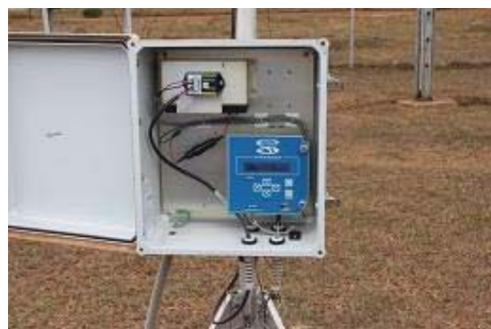
Sutron datalogger and power unit
