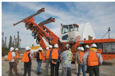
One of two Jumbos used for horizontal drilling in the transfer tunnel. Completely automated, these machines are equipped with three parallel arms that can bore up to six metres into the rock. Some 150 boreholes per blast are required to form the arch of the tunnel.
