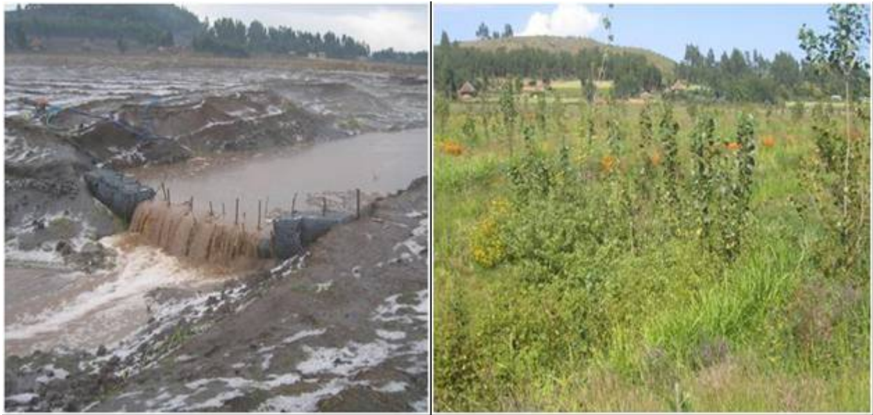
Plate 7. A gabion check-dam filled with soil (top and bottom plates) and its effect after one year
