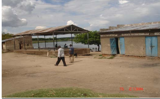
Plate 4.5.4: Poor state of fishing washing canopy, slab and stores at Katwe Fish Landing Site, Lake Edward Uganda
