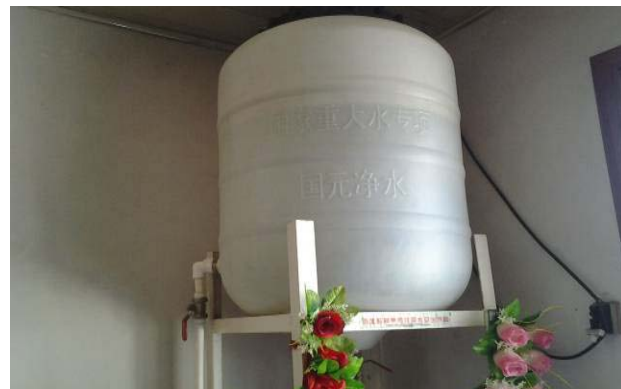
Drinking water tank
