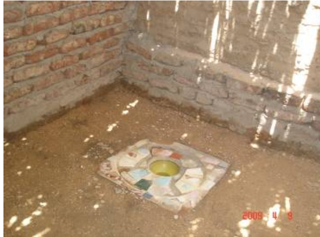
Plate (7): the latrines connected to the unit
