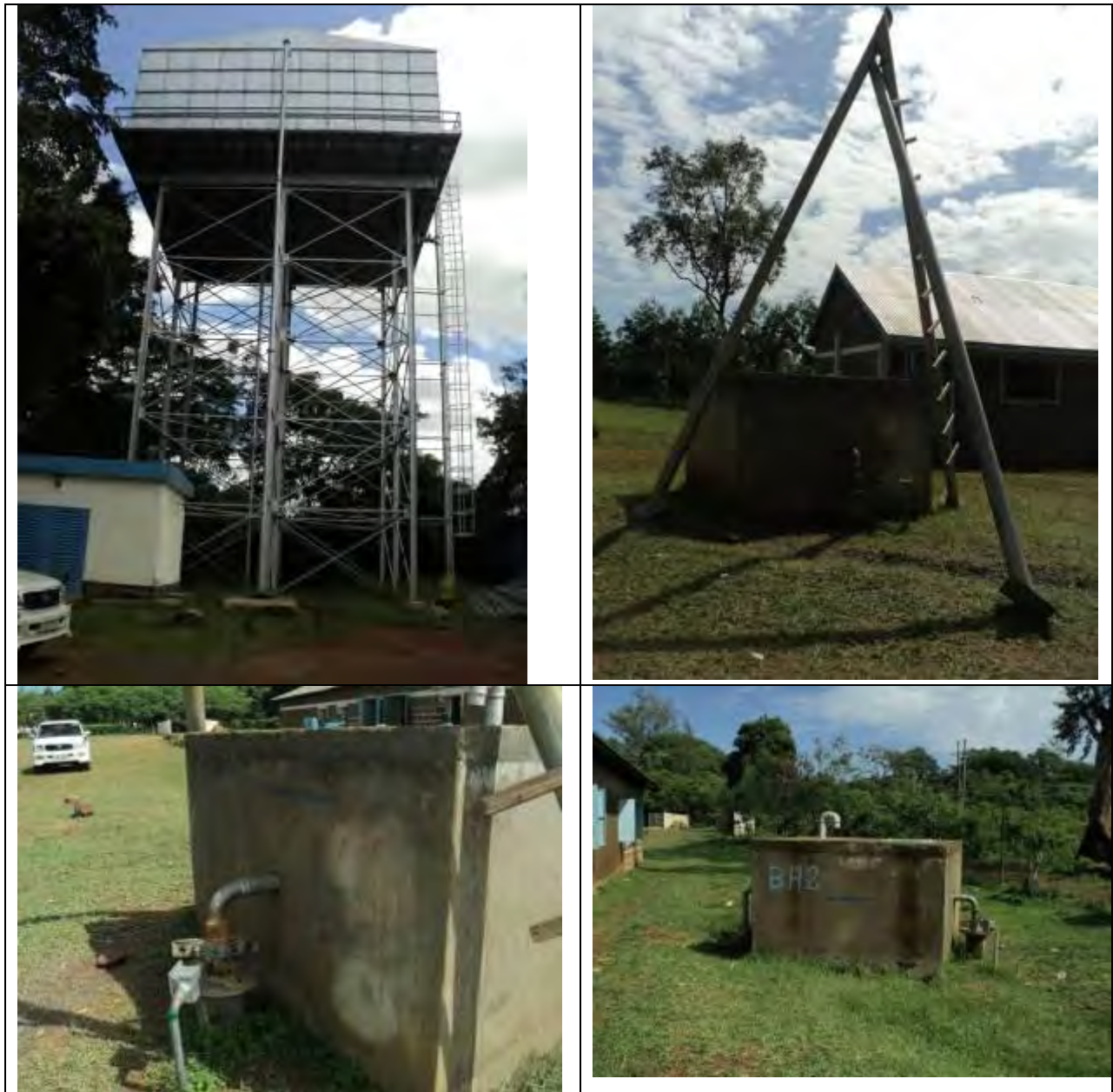
Figure 6-19: Nambale Water Supply System based on motorised boreholes
