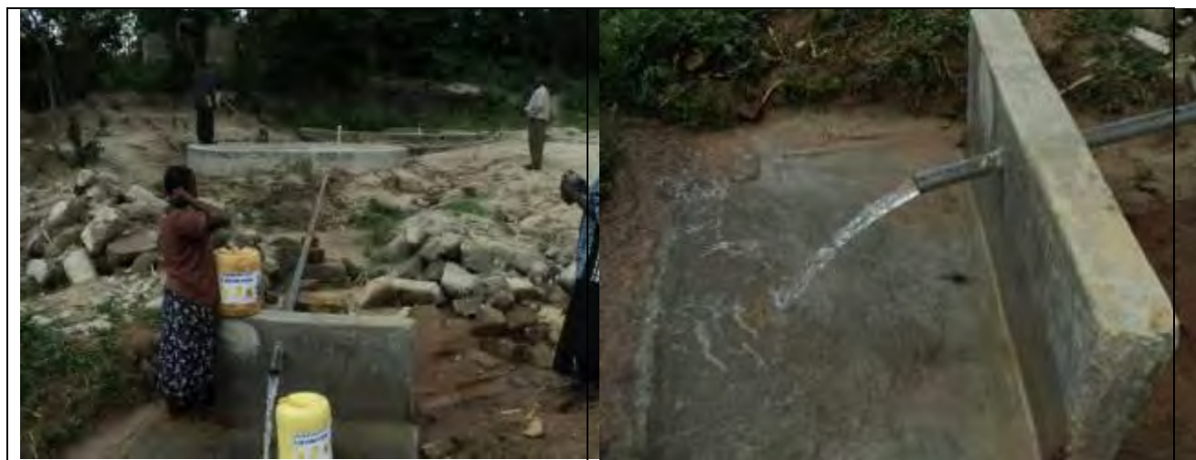
Figure 6-20: Namasale water supply system based on a protected spring
