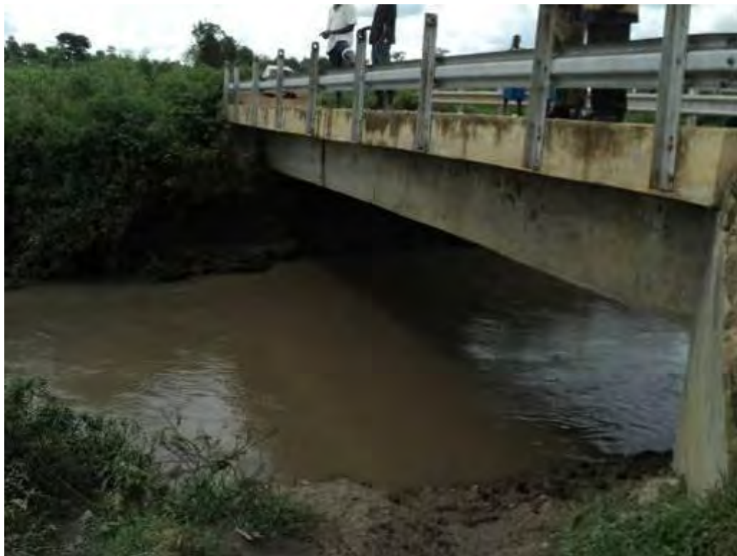
Figure 6-24: Heavy siltation in Namanderema River
