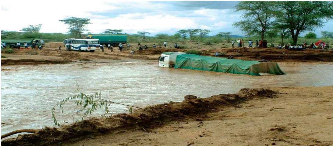
Photo 3: A flooded road section in Kenya
