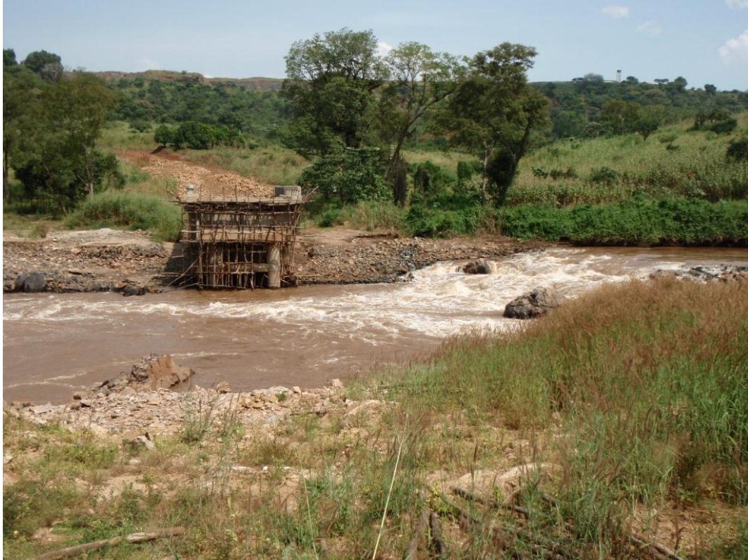
Plate 5. New bridge under construction on the Didessa River. Will provide much needed link to project area from main road and markets.
