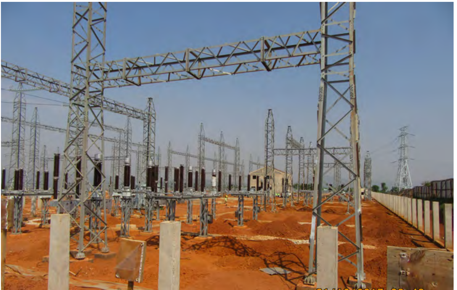
Shango Power Sub-Station in Rwanda.
