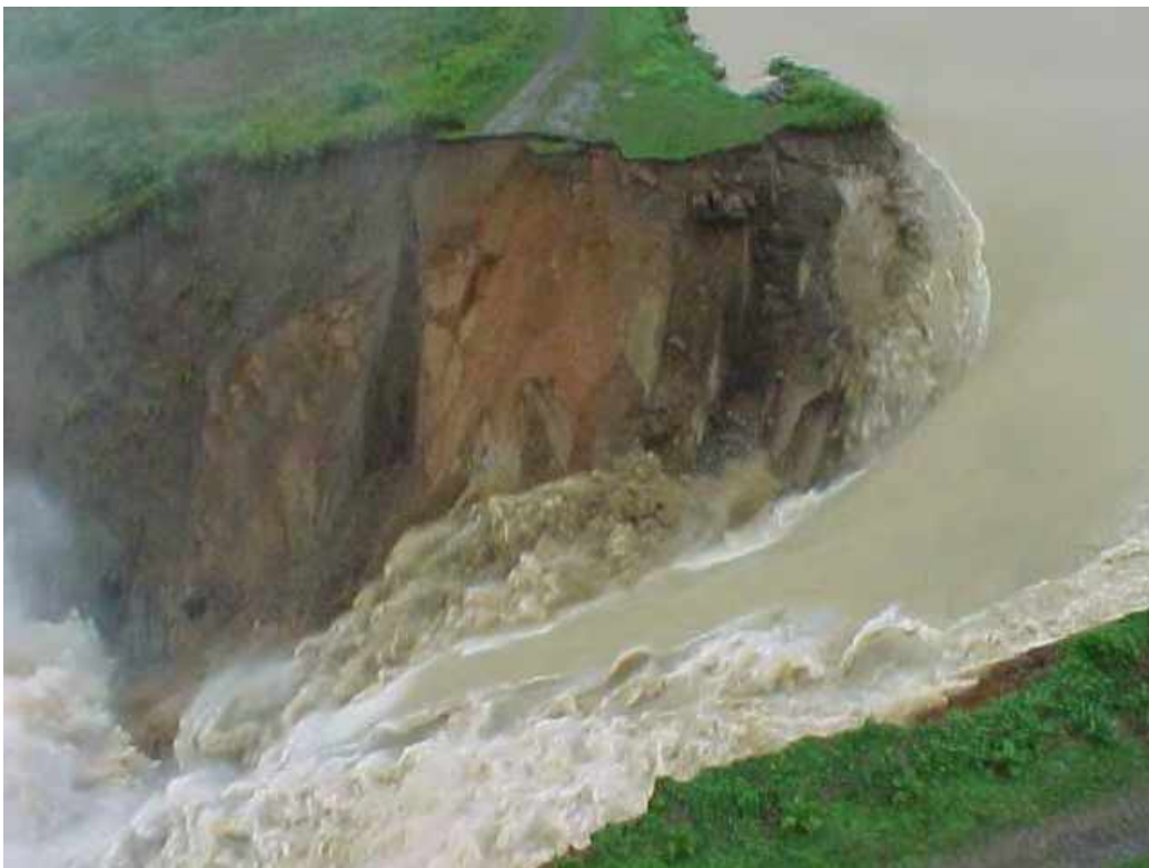
Figure 16: Headcutting Progressed to Reservoir
