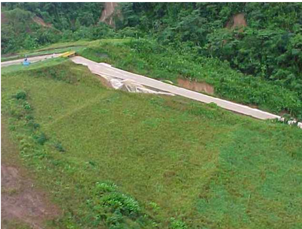
Figure 14: Overtopping Along Entire Length of Chute
