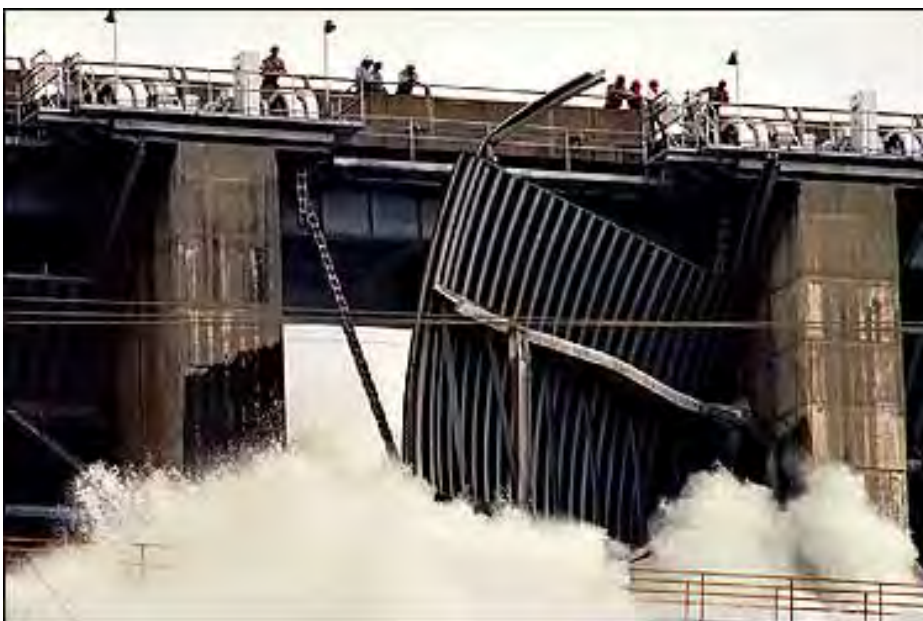
Figure 39: Folsom Dam radial gate failure
