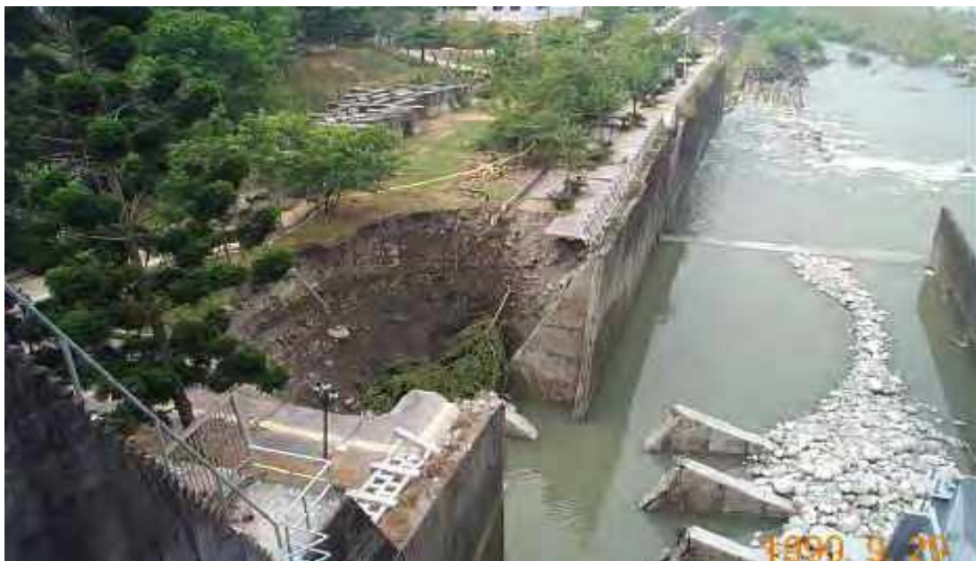
Figure 12: Failed Spillway Wall at Shih-Kang Dam
