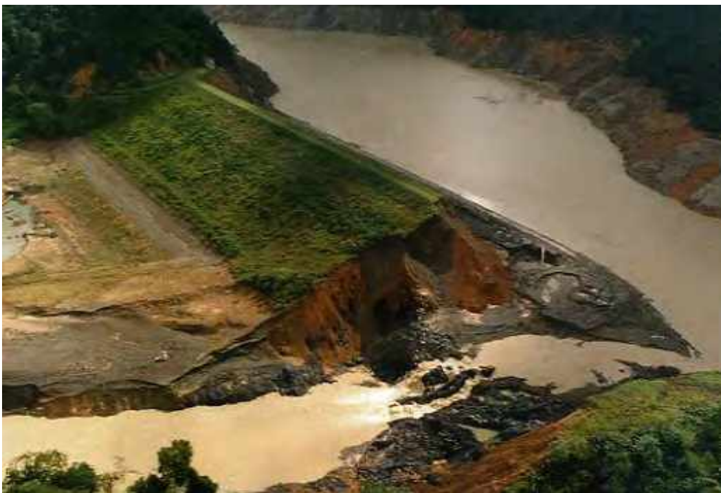
Figure 18: Aftermath of Reservoir Breach
