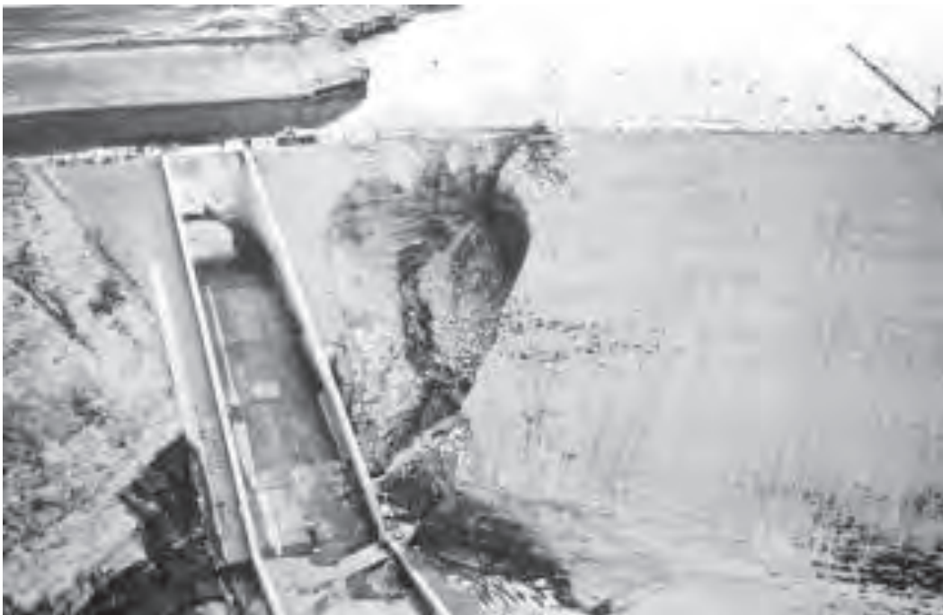
Figure 8: View of the piping at Fontenelle Dam
