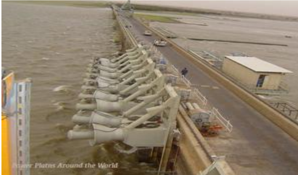
Figure 6 Matrix Turbines installed in Jebel Aulia Dam(Source Hydro Matrix)
