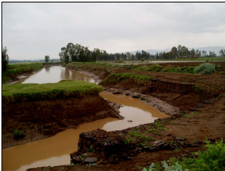
Figure 4-7: Gabion Retaining Wall on Ribb River Upstream of the Main Bridge Site
