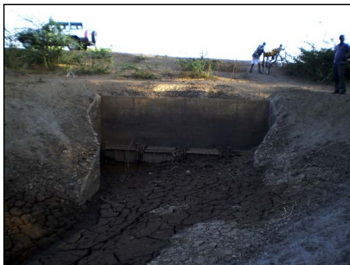
Figure 5-1: Outlet of Drainage Outfall with Flap Gate at Amibara Irrigation Project (Source: Consultant's Private Library 2007)
