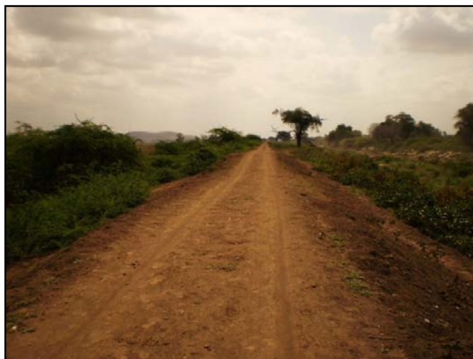
Figure 3-1: Flood Protection Embankment at Amibara Irrigation Project Awash River (Source: Consultant's Library 2007)
