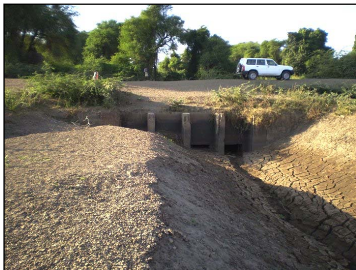
Figure 5-2: Sediment Deposition at the Inlet of Drainage Outfall Structure (Source: Consultant's Private Library 2007)
