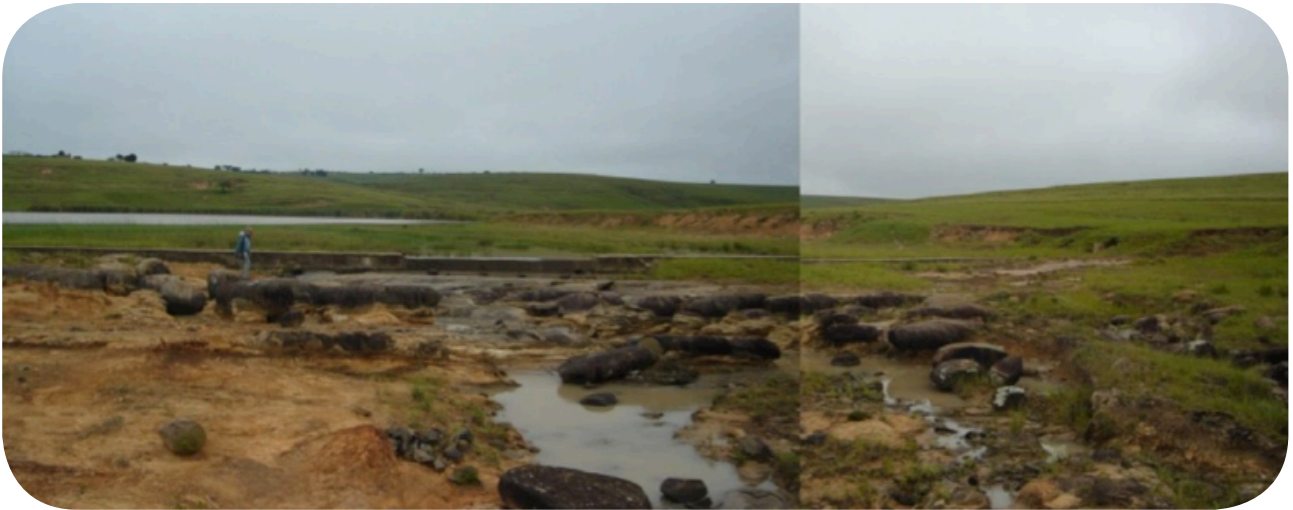
Figure 9.2 1: Backward erosion of the by-wash spillway of toleni dam in south africa
