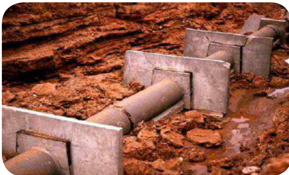
Figure 7.5 3: Pipe with intact anti-seepage collars shortly after failure of a small dam (mccook/2004).
