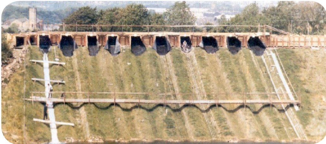
Figure 9.3 4: Testing under way on the left-hand of the ten channels at jackhouse reservoir near blackburn, uk
