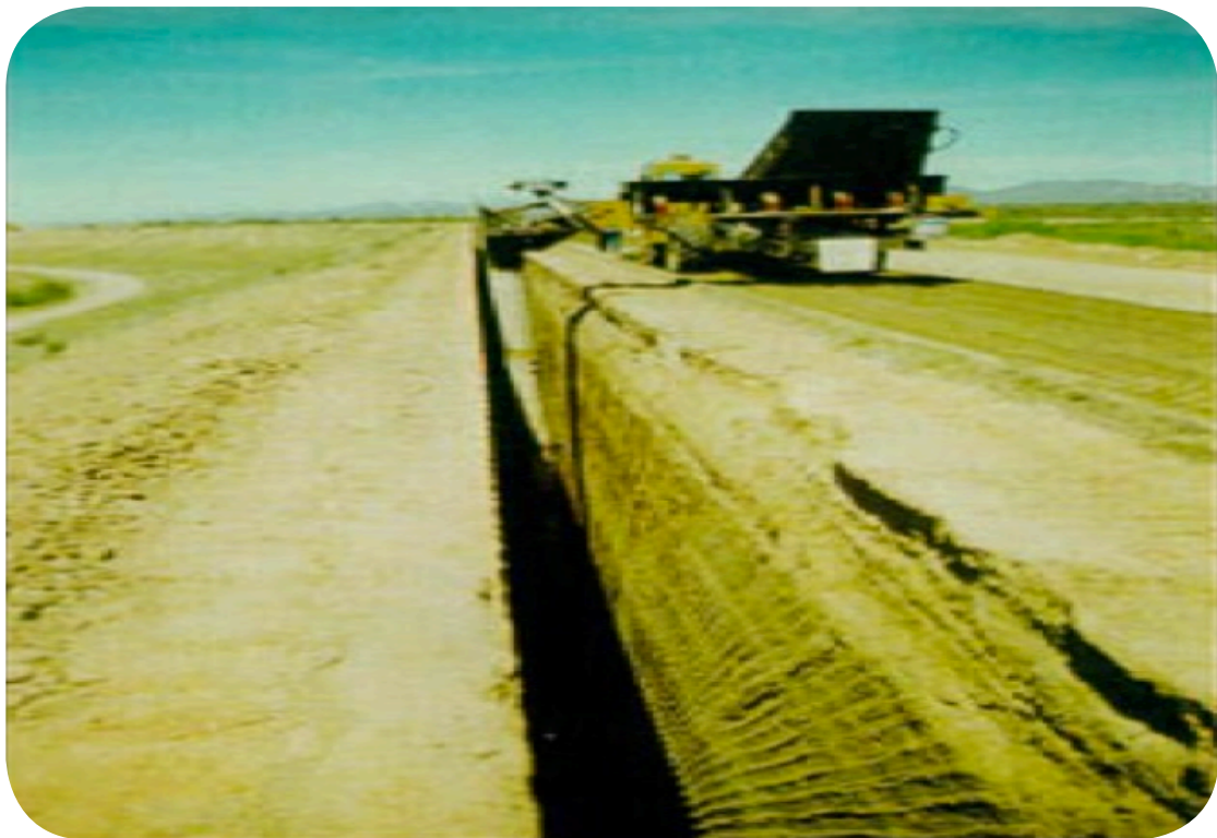
Figure 9.3 13: Central sand filter installed by open trenching from the crest of an existing low-height flood control dam in southwestern usa
