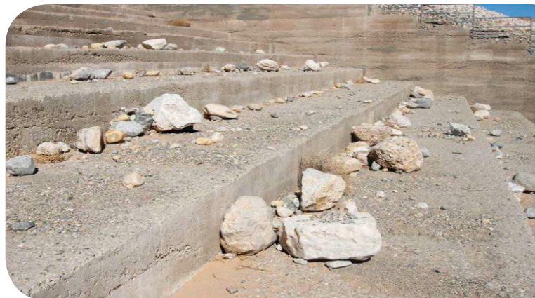
Figure 9.3 10 Boulders deposited on the rcc steps during 2005 storm (abdo and adaska, 2007)
