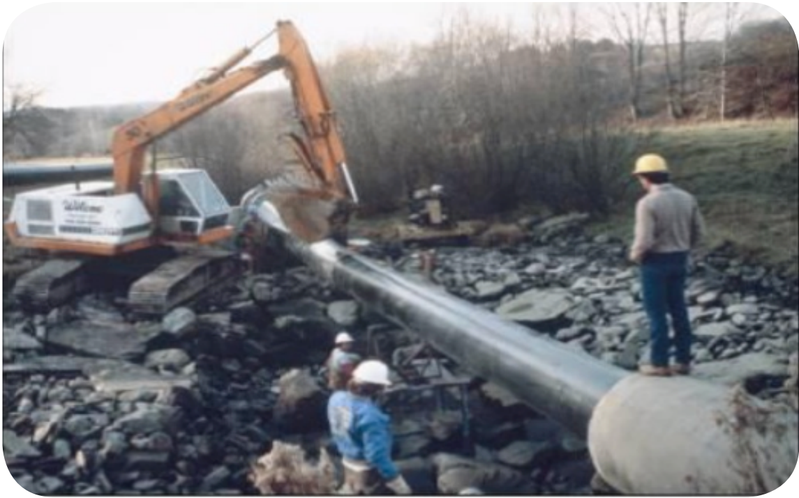
Figure 9.3 15: Example of sliplining – insertion of plastic (high density polyethylene) pipe into larger diameter concrete pipe (from fema, 2005)
