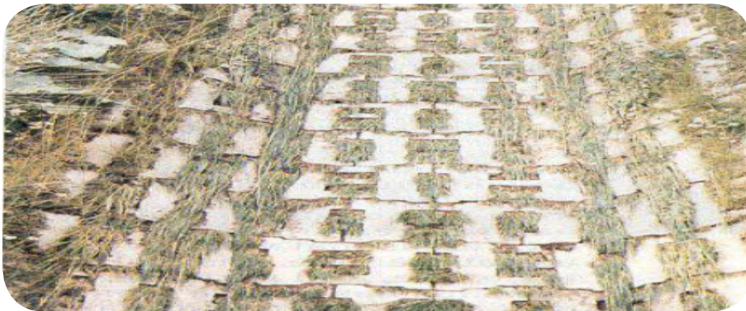
Figure 9.3 5: One of the cable-stayed block systems remains totally intact after a water test
