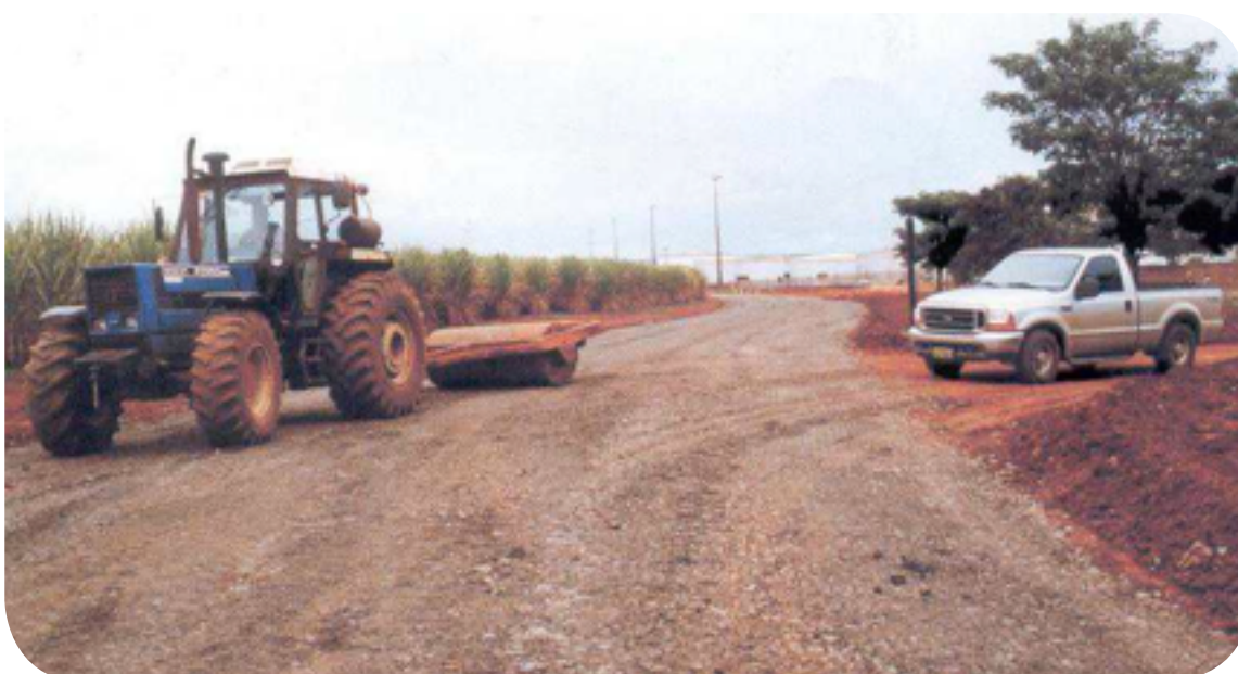
Figure 7.10 5: Constructing a rural road using a granular material composed by gneiss, limestone and bituminous shale.
