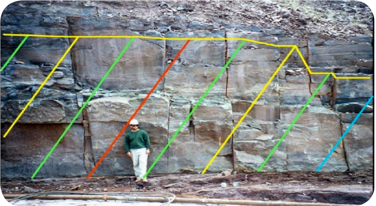
Figure 9.3 11: Vertical rock joints shown with angled grout hole orientation (Penn forrest dam rehabilitation, usa)
